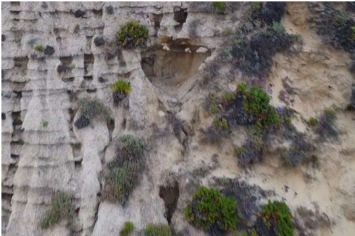
Photo 14: Screen shot of large and small erosion gullies below 255 Pacific Avenue provided by property owner drone footage (July 19, 2023).
